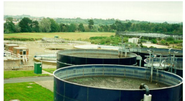
Sludge settlement tanks at a Sewage Treatment Works.
